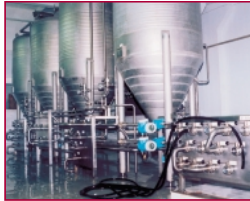
Automatic cleaning station (CIP) in ROSAR brewery
